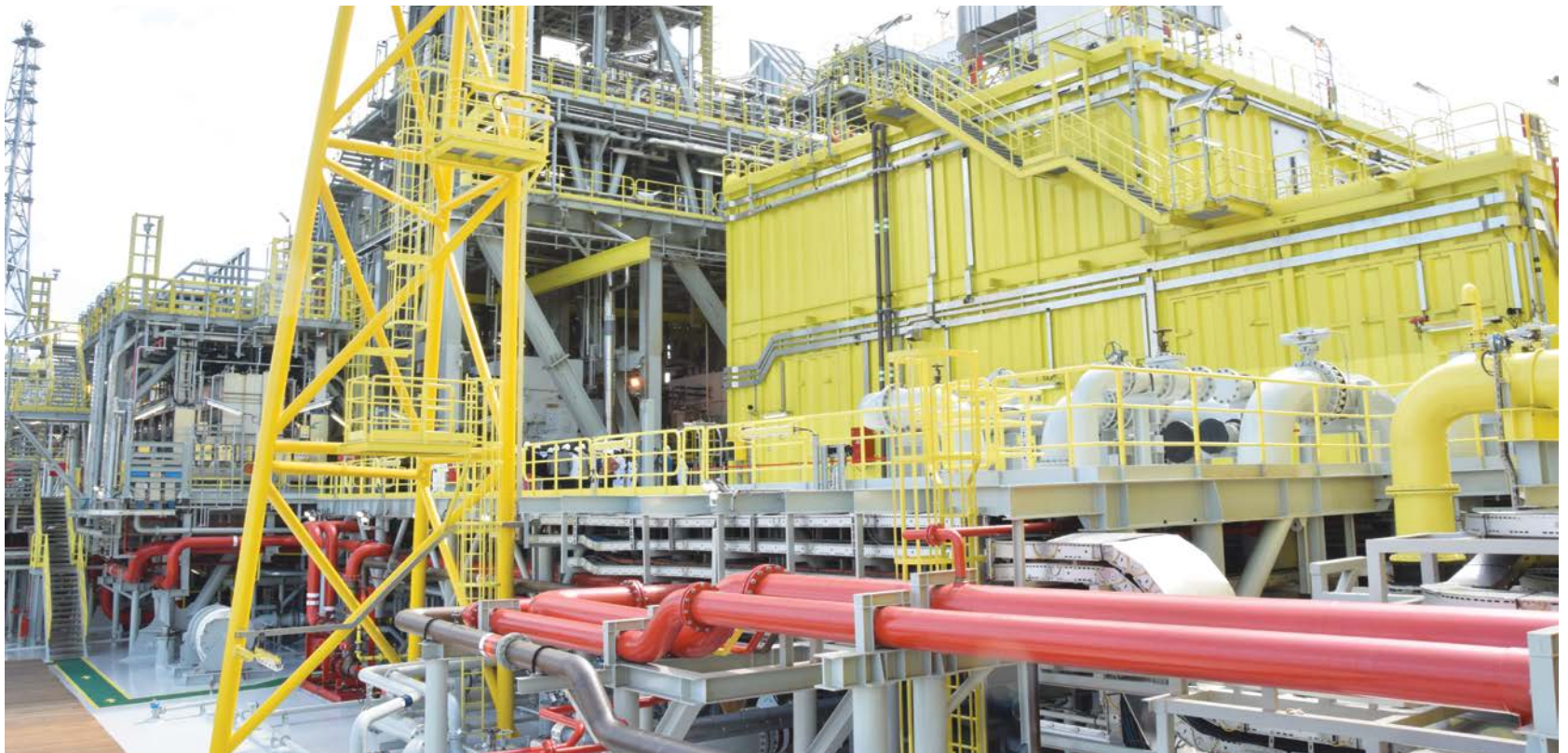
| Portside Area of FPSO showing the Fire Fighting main rings
